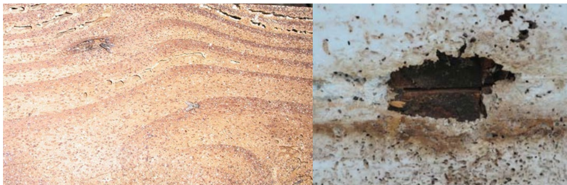
Image left – Damage of wooden pillar caused by burrowing larva. Photo from Cornell University Image right – Insulation damage by darkling beetles. Photo Robert Rowland
