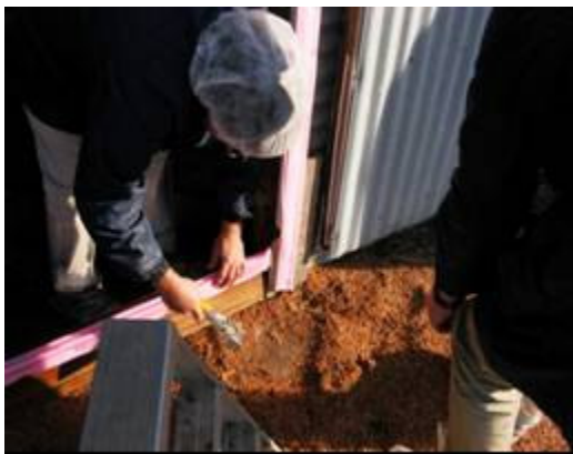
Photo 1: Install polystyrene tape weather-stripping around the perimeter of end doors to improve their seal.
