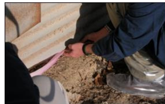
Photo 5: Polystyrene rope and tape can be used to seal air from entering between the wall metal and the foundation.
