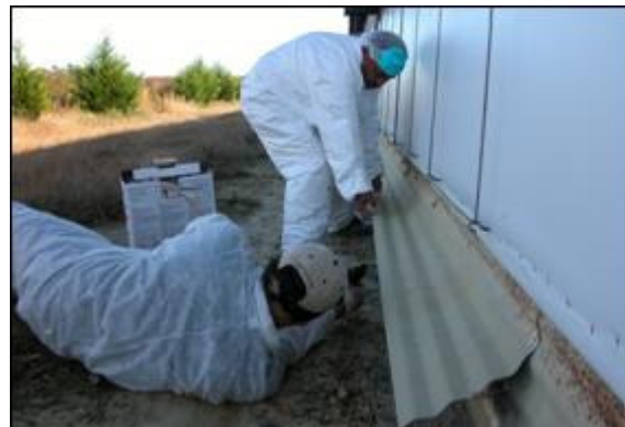
Photo 4: Spray foam being applied to fill the gap between the plate and top of the foundation.
