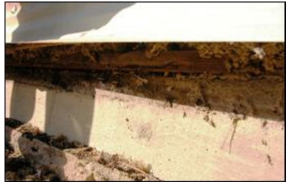
Photo 2: The gap between the top of the foundation and lower plate is a source of cold air leakage on birds and litter.
