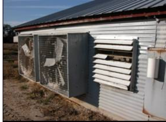
Photo 6: Replace broken fan shutter panels. Don't leave a permanent hole for cold air to enter the house
