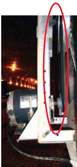
Figure 7. This fan motor and pulley are being pulled upward because of poor support on the fan frame.
